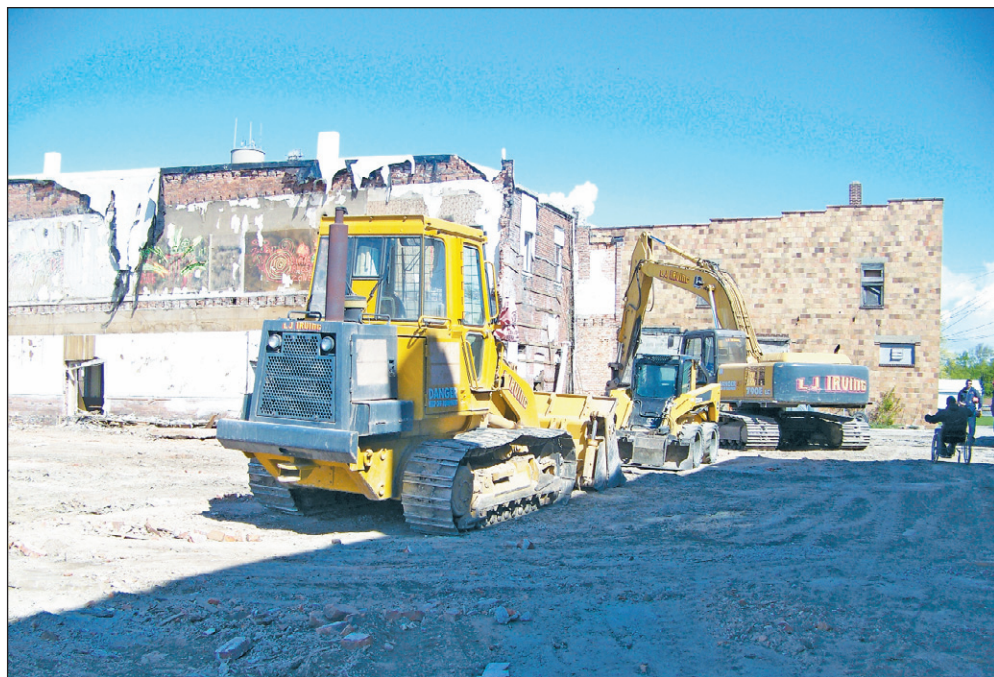
The final portion of demolition in downtown Payne was occurring earlier this week in order to make way for the construction of a new Antwerp Exchange Bank at the corner of Merrin and Main Streets. Town officials anticipate that final demolition and cleanup should be completed by the end of this week.
